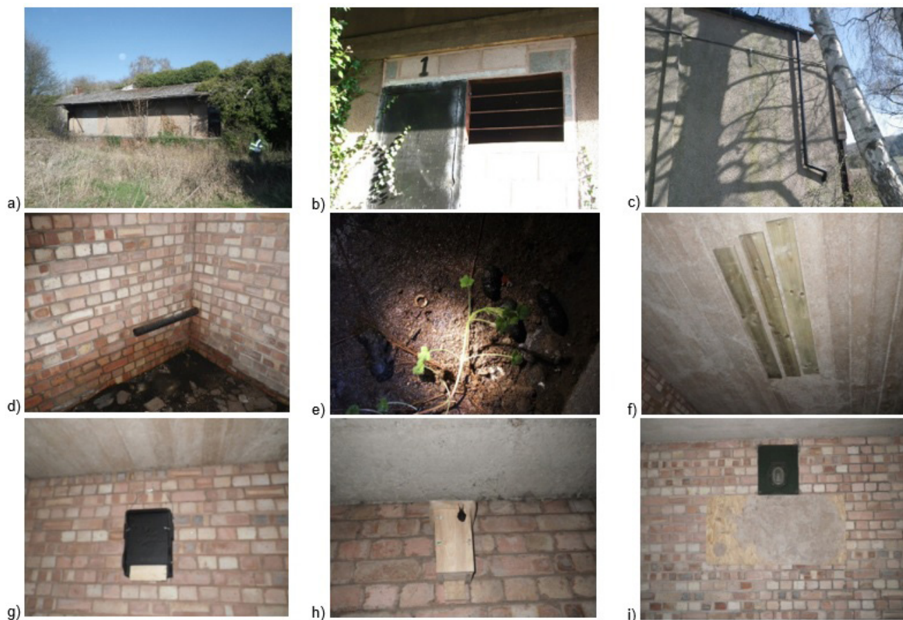
Fig. 3 – Magazine bat enhancement photographs. These comprise: a) general view showing blocked door, b) grille and door, c) external pipework diverted internally, d) internal pipework, e) wet floor (and barn owl pellets) underneath Magazine 2 grille, f) rough untreated timber on ceiling, g) internal Schwegler 1FF bat box, h) internal wooden bat box, and i) internal rough wooden boarding (beneath historic light fitting panel).
